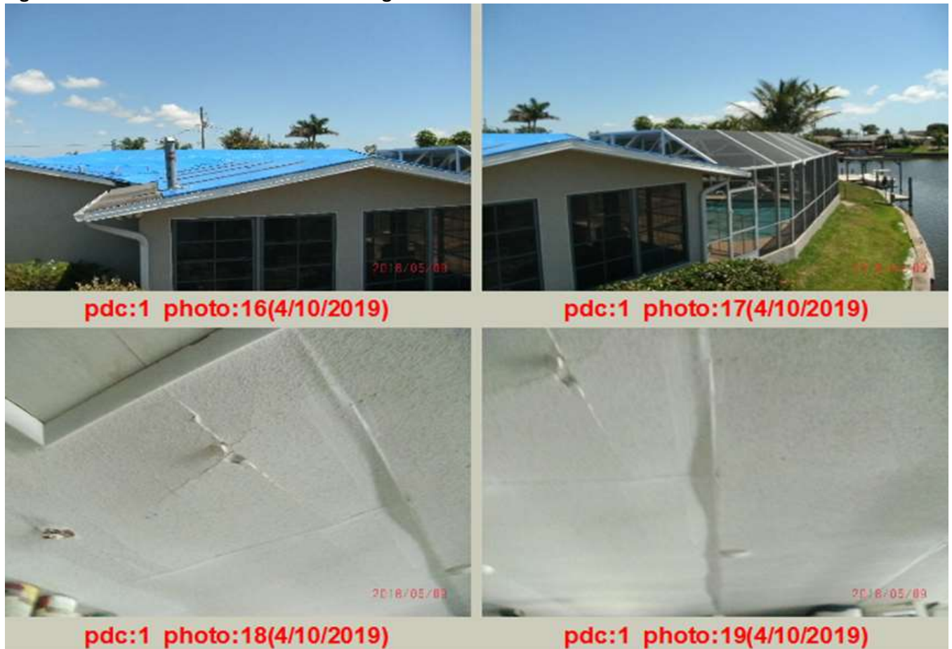
Figure 9-7.1 SFR with Hurricane Roof Damage
